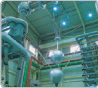
High Voltage Test / Impulse Test
